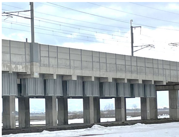
Experimentally installed sound-absorbing panels
