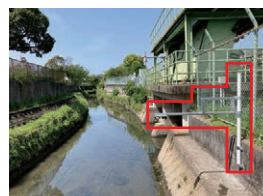
Example of IoT water level sensor installation (Neyagawa, Osaka)
